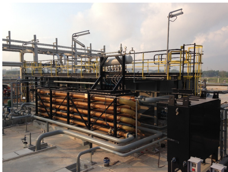
CPR as part of a refinery waste water treatment plant. The material of construction is GRE-CST (conductive)
