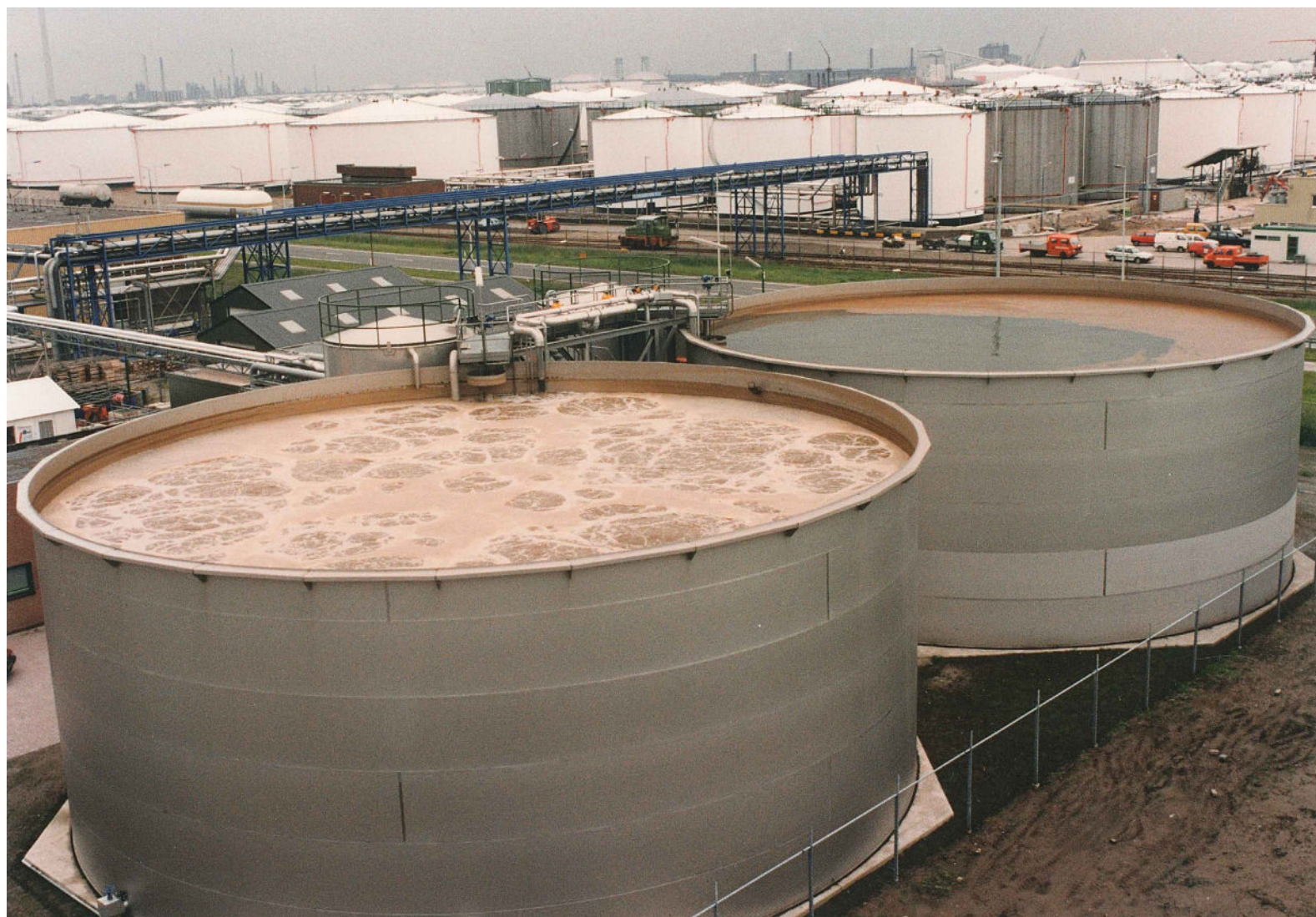
Picture 2: Sequencing Batch Reactor biological wastewater treatment plant
